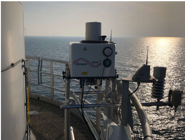
Figure 2. Long-range-scanning lidar and additional measurement systems (on the right side) on the TP of one of the northernmost wind turbines (K01) at the wind farm Gode Wind 1.
